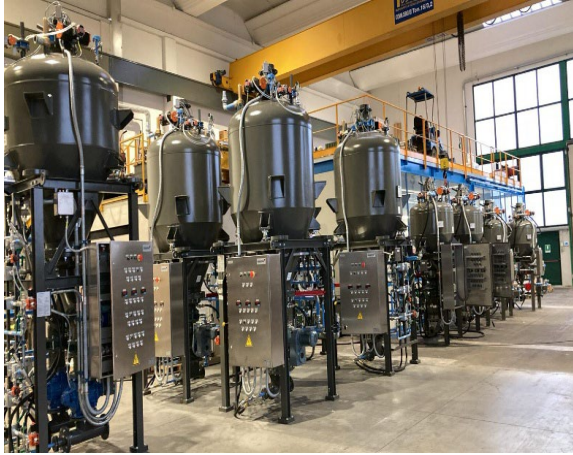
Injection System Vessels
